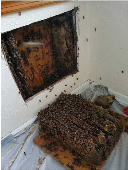
Figure 13. Creating access to a honey bee colony nesting in a wall. Credits: Jason Deeringer, Bee Serious Bee Removal, LLC
